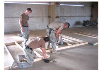
(Above) C/4-31 IN Soldiers begin to build living quarters for themselves at PB Dragon
